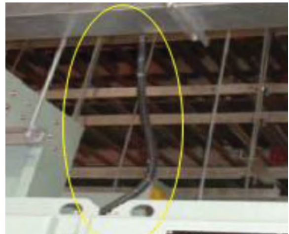
Flexible conduit protecting FO sensing cable
