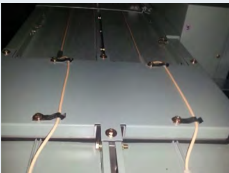
FO sensor cable fixed in place using busbar manufacturer-supplied clip.
