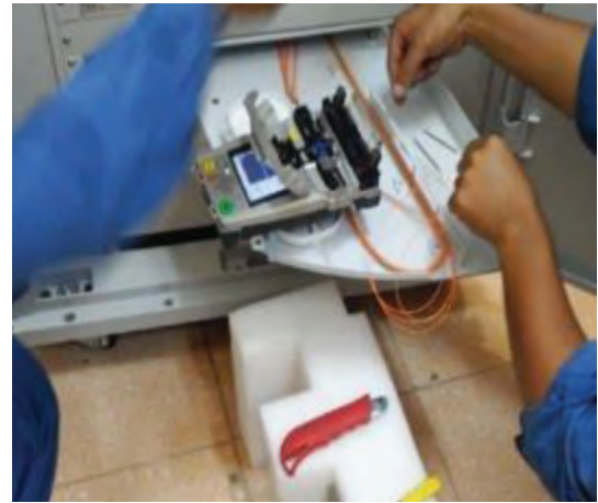
Managing fiber on a splice tray
