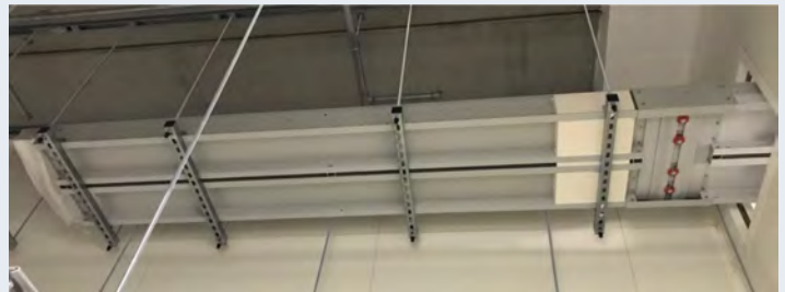
Busbar with fire barrier crossing partition wall (without penetration seal)
